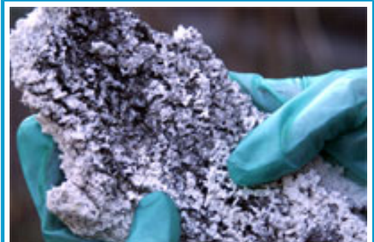
[Mold growing on a piece of ceiling tile]
